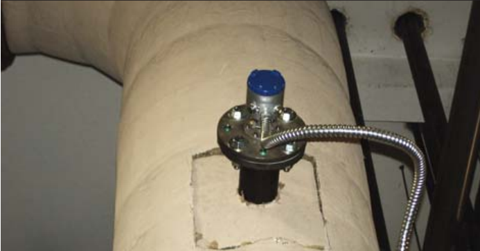
ZP-O2 Detector and Probe mounted in the stack.
