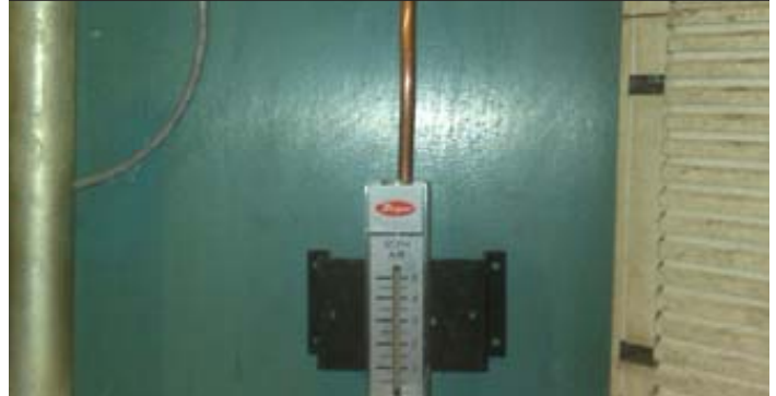
Flow meter tubed to the O2 Detector
