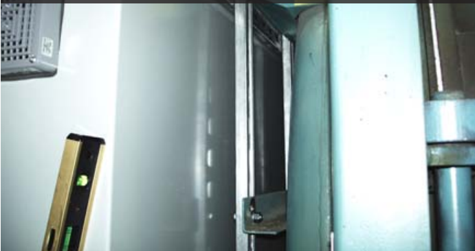
New BurnerMate Universal panel bolted to uni-strut frame.
